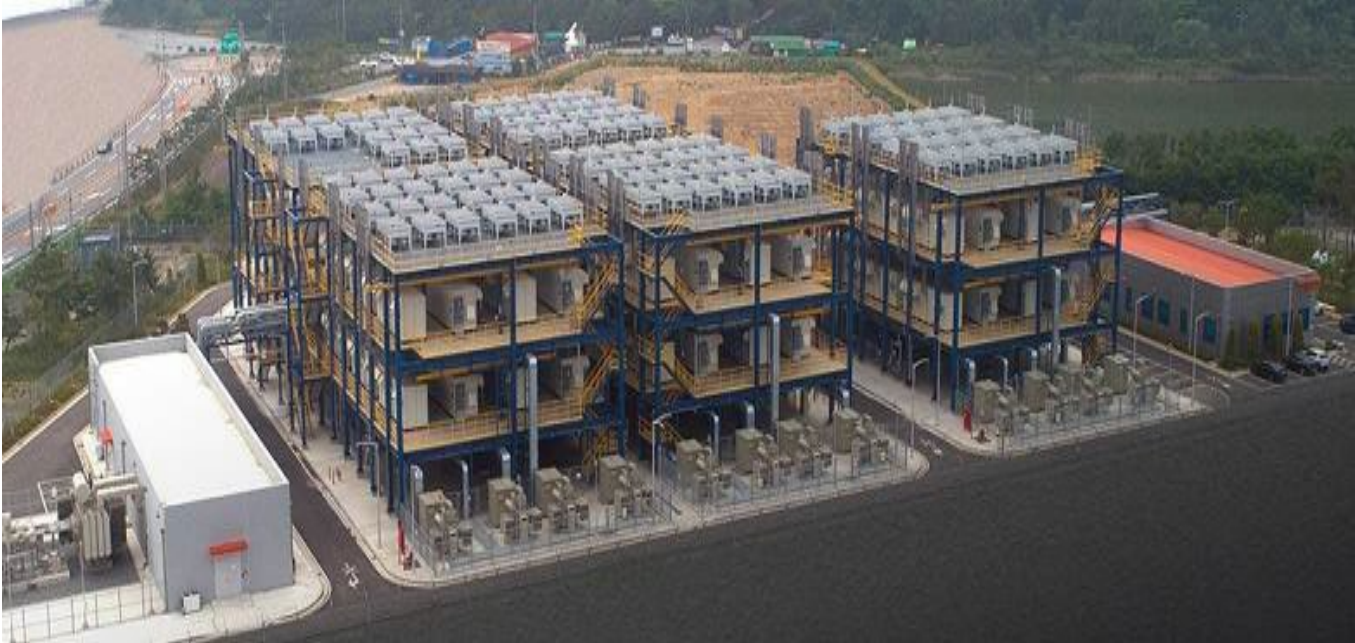
Daesan Industrial Complex in Seosan, South Korea (50MW, multi-story 114 unit Installation)
